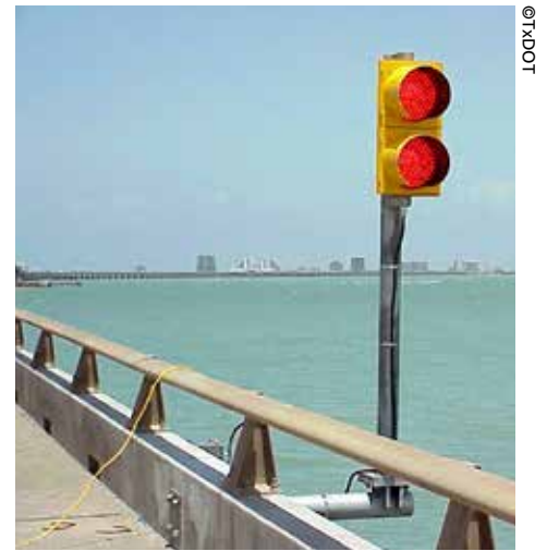
The Collapse Warning System on the Queen Isabella Causeway in Texas includes flashing red traffic signals.
