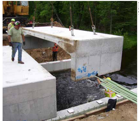
The mid-section of the precast superstructure for a bridge on M-115 is placed as part of the Michigan Department of Transportation’s performance contracting project.
