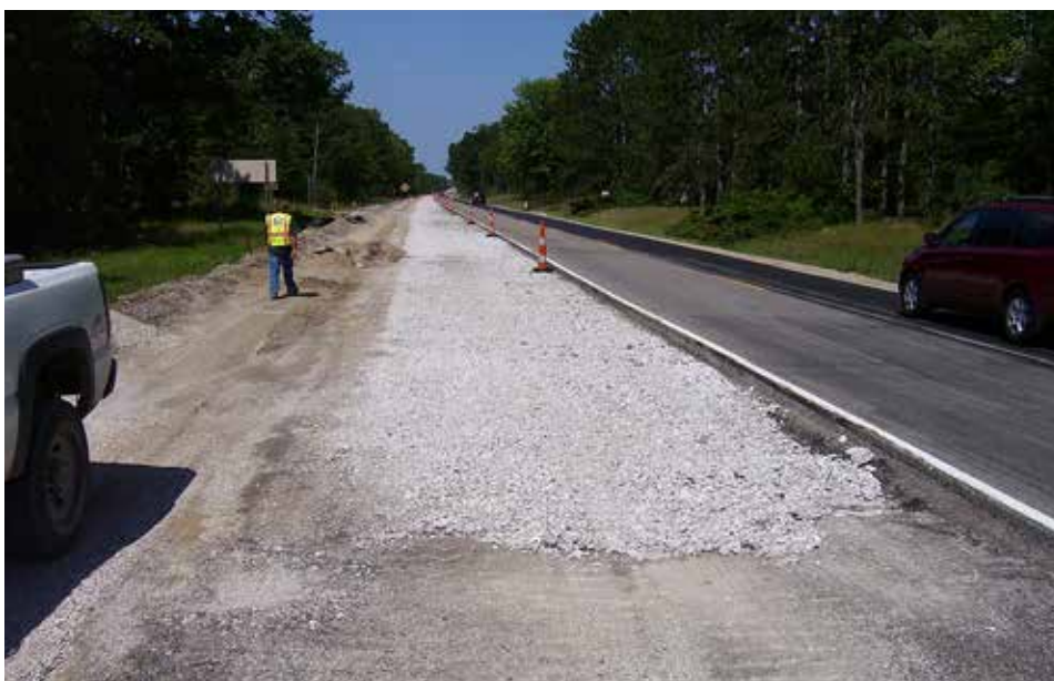
Using performance contracting, the Michigan Department of Transportation rehabilitated an 8.9-km (5.56-mi) stretch of M-115 in Clare County.
