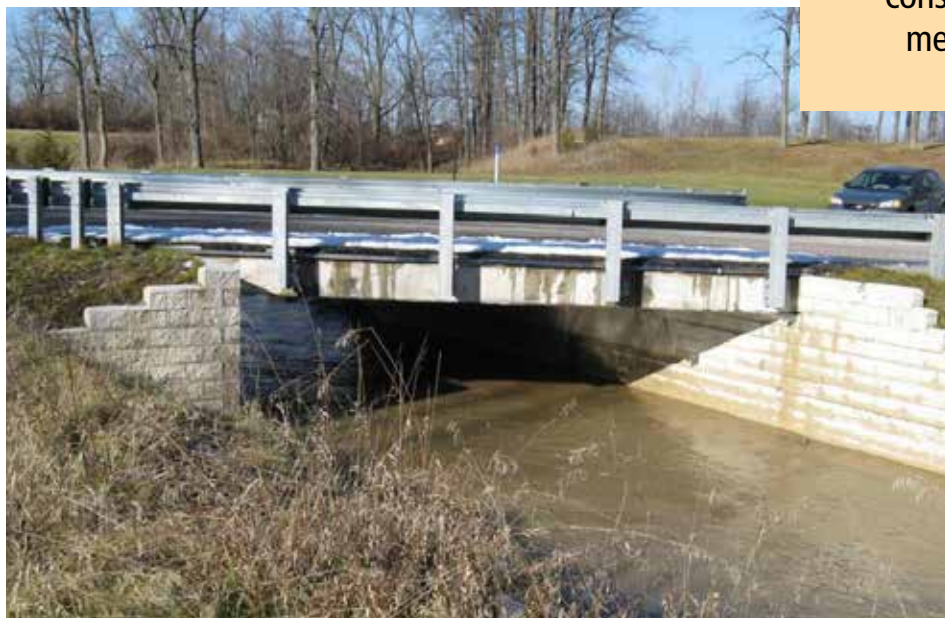
Bridges built using the Geosynthetic Reinforced Soil Integrated Bridge System (GRS-IBS) include the Vine Street Bridge in Defiance County, OH.
