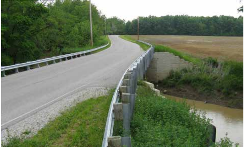
The Bowman Road Bridge in Defiance County, OH, was the first bridge in the world to use GRS-IBS.
