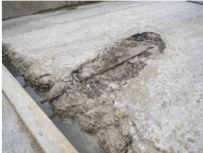
Figure 8. Distressed region on the westbound lane near the western abutment: test region B1. (2)
