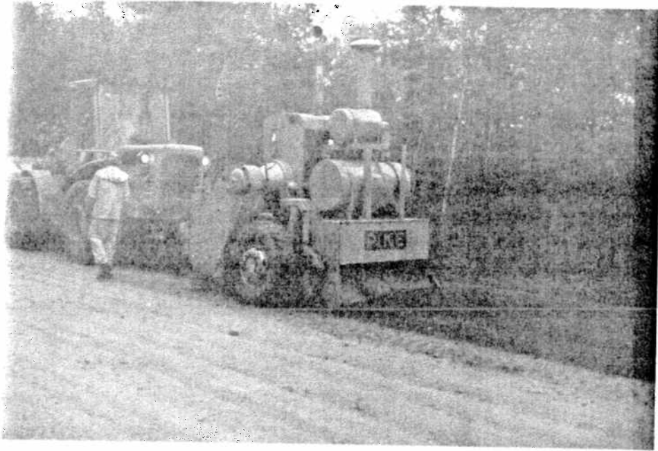
FIGURE J-15: Hammermilling Operation
