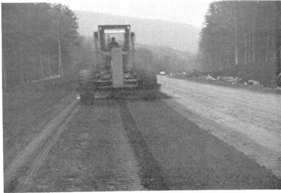
FIGURE J-17: Pulverized Material Graded to Required Depth, Prior to Compaction (Looking South)
