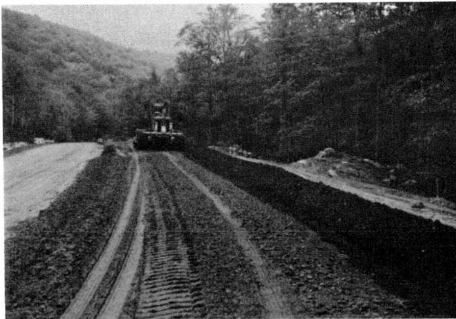
FIGURE J-10: Grader Windrowing Portion of Material to Extreme Outside (Looking North)
