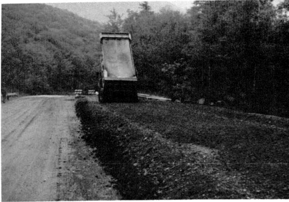
FIGURE J-9: Crushed Gravel Being Applied Directly on Reclaimed Material (Looking North)
