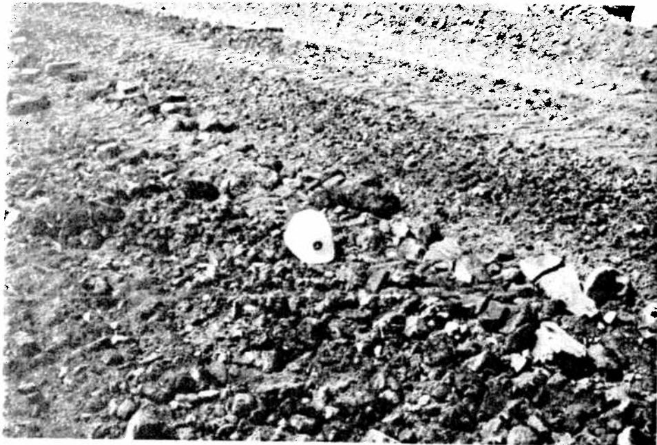
FIGURE J-5: Existing Pavement Crushed; Background, After 5 to 6 Passes of Rotating Mill; Foreground, After 2 to 3 Passes of Rotating Mill
