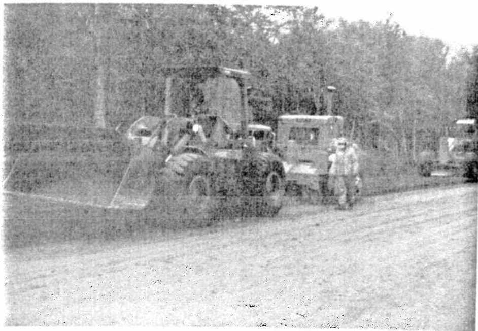
FIGURE J-16: Hammermilling Operation
