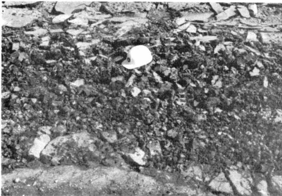
FIGURE T-4: Existing Pavement After Ripping and Approximately Eight Passes of the Rotating Mill
