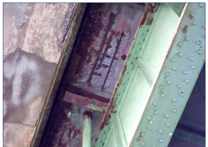
Figure 6. Photo. UAS image of deterioration between steel girders and spandrel arches.
