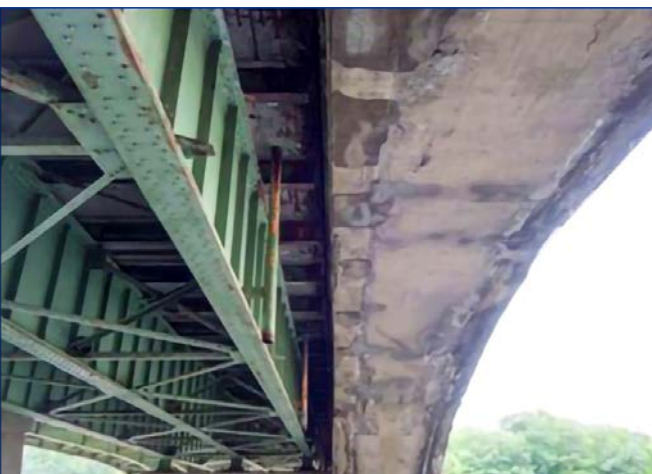
Figure 5. Photo. UAS image of space between spandrel arches and primary bridge structure.
