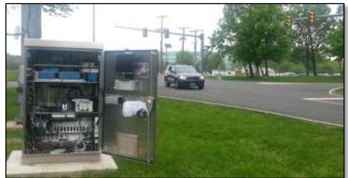
Intelligent intersection and signal controller cabinet at TFHRC
