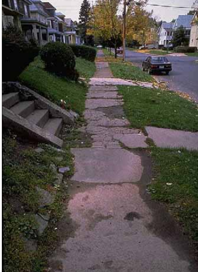
Figure 7-1. Photo. Inadequate maintenance of sidewalks makes a short walk difficult to maneuver.
