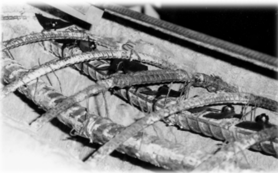
A close up of the defect showing the exposed rebar bending at the onset of failure. The steel balls attached to the rebar were targets for the NDE team's laser device that provided useful information about the bending of the rebar.
