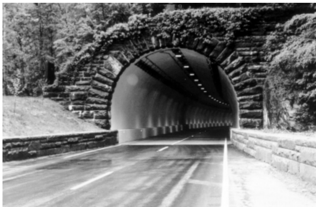
Water in tunnels often freezes because it doesn't have the chance to drain.
