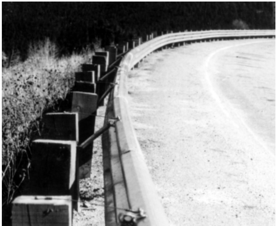
Installing, repairing, upgrading, and replacing roadside hardware such as this guardrail requires hundreds of millions of dollars annually.
