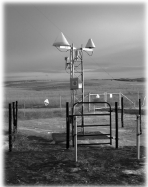
FHWA NDGPS site at Whitney, NE, equipped with NOAA surface meteorological sensors. Shared use of Government resources saves both time and money.
