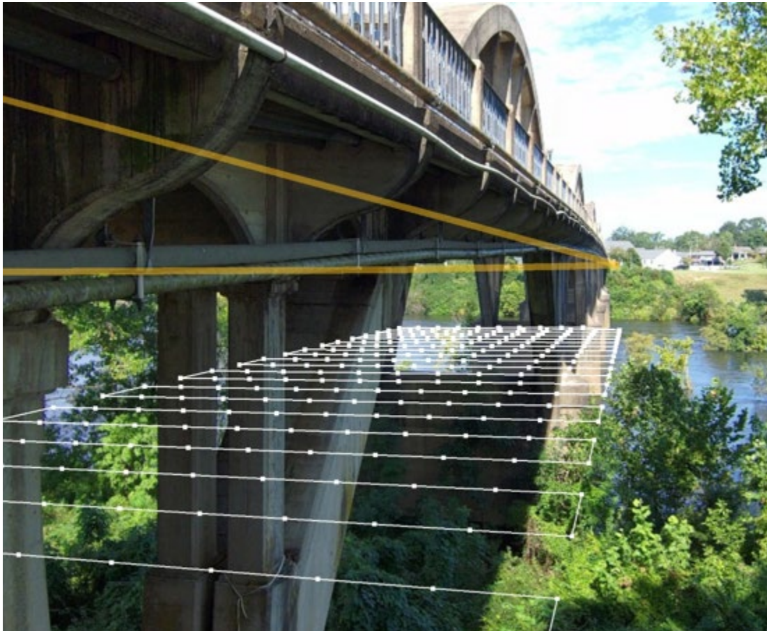
Figure 6. UAS software allows for pre-mission planning prior to the bridge inspection.(Source: ALDOT)
