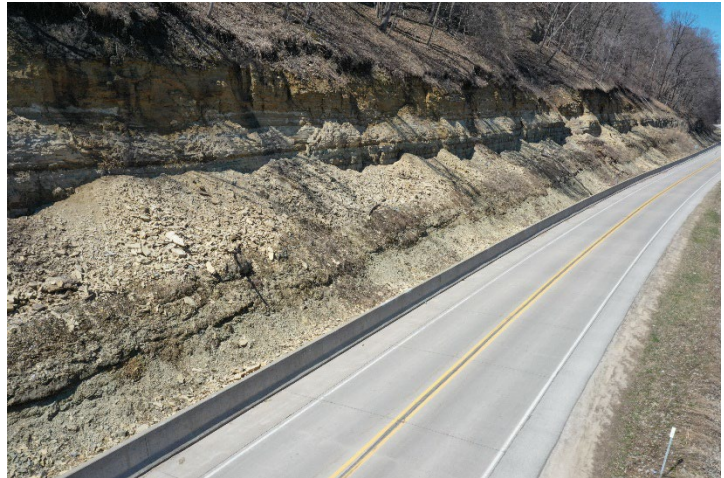
Figure 3 - UAS Imagery of Rockfall (Image Courtesy Iowa DOT)
