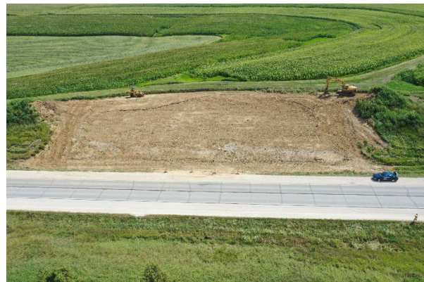
Figure 2 - UAS Imagery of Earth Movement (Image: Iowa DOT)
