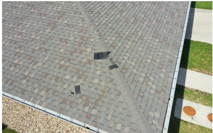
Figure 4 - UAS Imagery of Wind Damage on Iowa DOT Building (Image Courtesy Iowa DOT)
