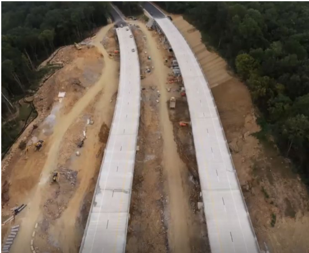
Figure 6. Still-capture of UAS-Collected Images Creating a 3D Experience of an Ongoing Project (Source: Alabama DOT)
