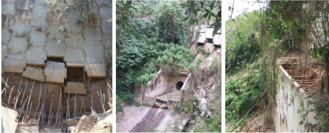
Figure 2. Use of UAS for Data Gathering of Three Assets in One Site. (Source: Puerto Rico DTPW)
