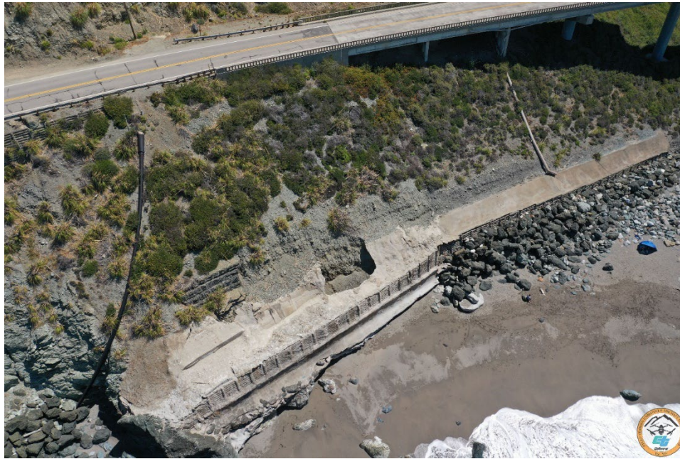
Figure 4. Lime Kiln Bridge on Highway 1 on the Big Sur Coast (Photo courtesy of Caltrans Steep Terrain UAS Group)
