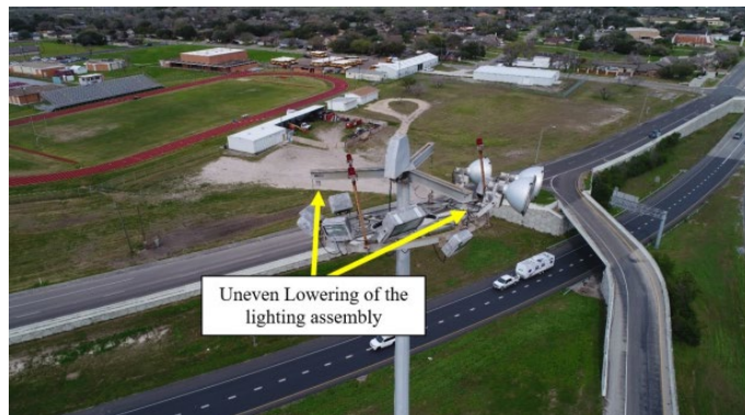
Figure 2. UAS Image of HMLP Lighting Assembly. Source: TxDOT
