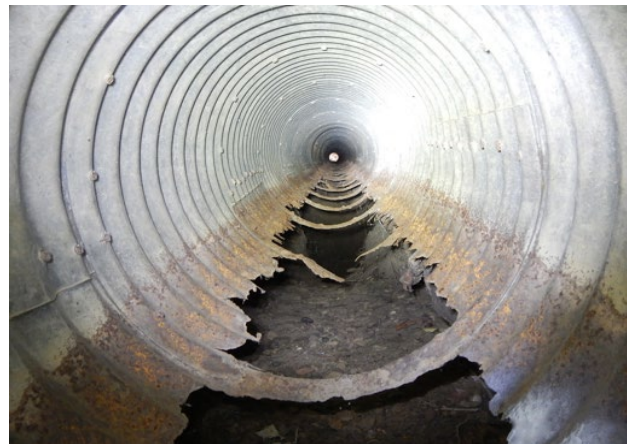
Figure 4. UAS Inspection of Deteriorated Culvert. Source: ODOT
