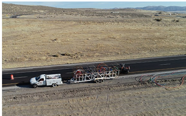
Fiber conduit being installed along I-84 in Box Elder County, Utah. Photo: UDOT
