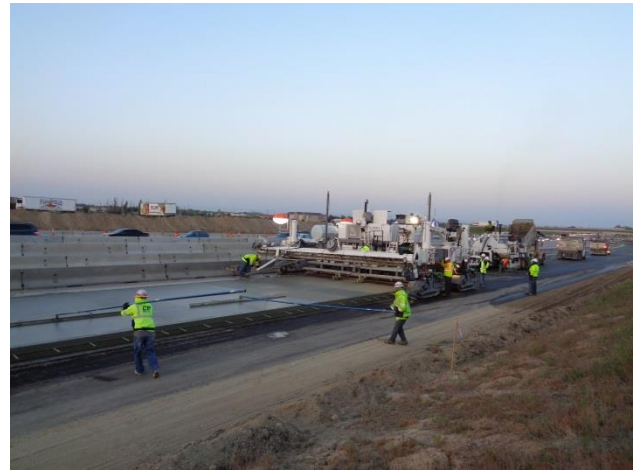
Figure 4. Use of a Final Finisher (auto-float) and Hand Finishing Behind the Paver
